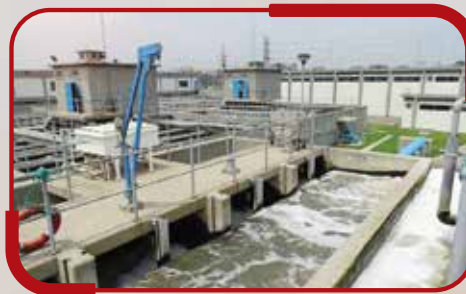
Gandharbpur Water Treatment Plant
