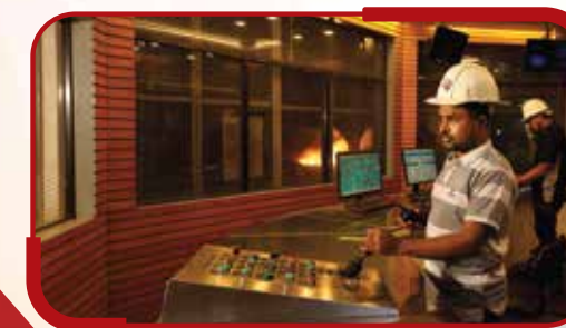
ROLLING MILL CONTROL ROOM
